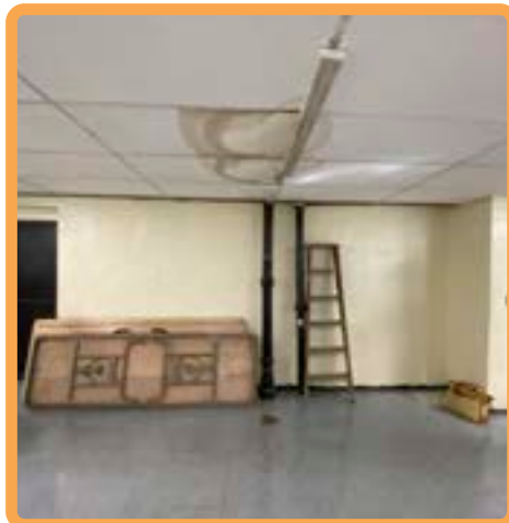
05: Water damage evident on ceiling tiles
