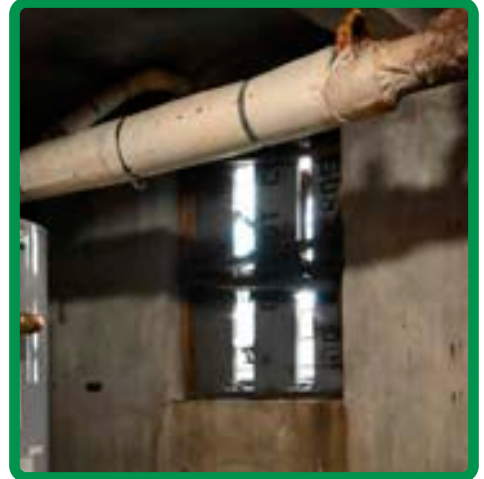
03: Missing window in hot water storage tank room
