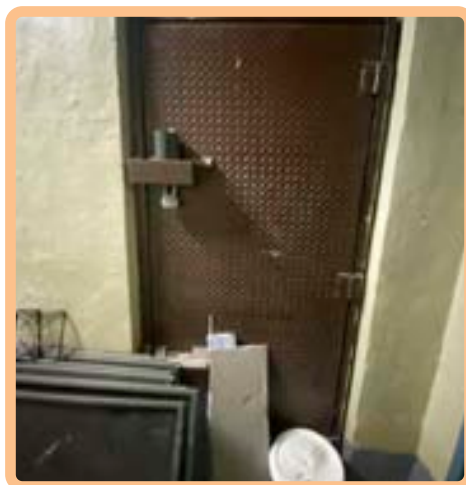
08: Locked and blocked metal door to community room
