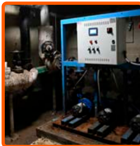
05: Water intake system
