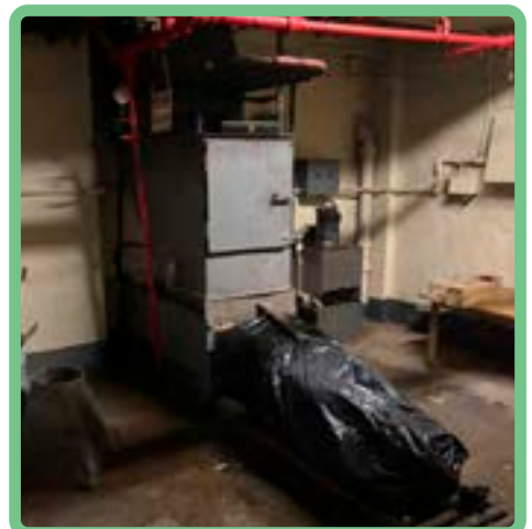
09: Waste compactor room
