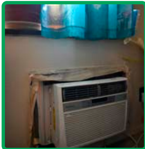
05: Resident provided AC unit
