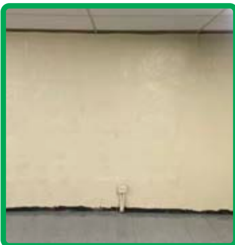
07: Non-functional outlet on wall
