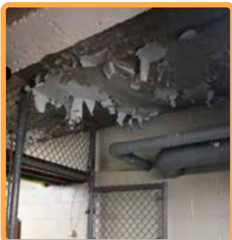
07: Water damage and appearance of mold in Office
