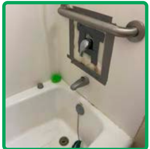
06: Leaks patched with tape and plastic by Maintenance
