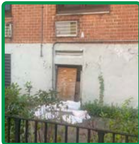
08: Missing window to cellar
