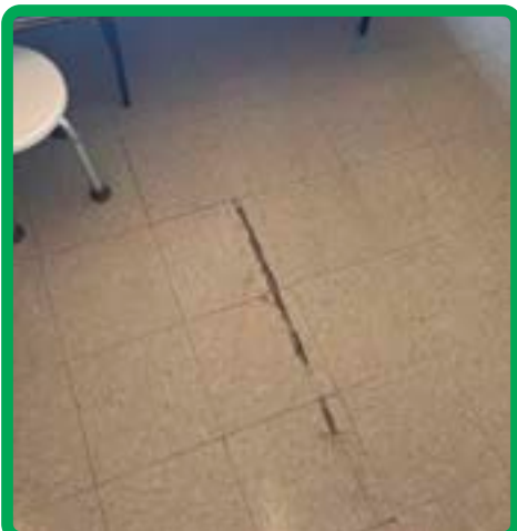
07: Damaged floor tiles
