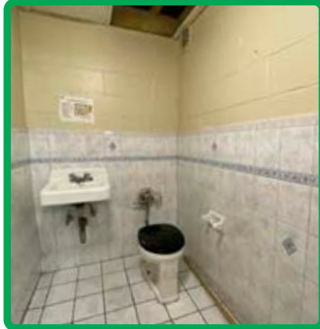
02: Restroom in Community Space w/ missing ceiling tile
