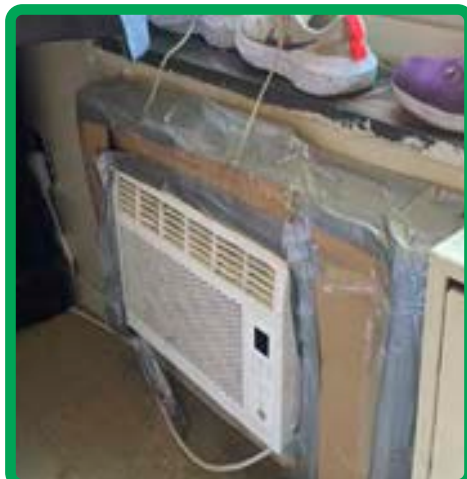
08: Ill fitting AC unit creates thermal breaks in exterior walls
