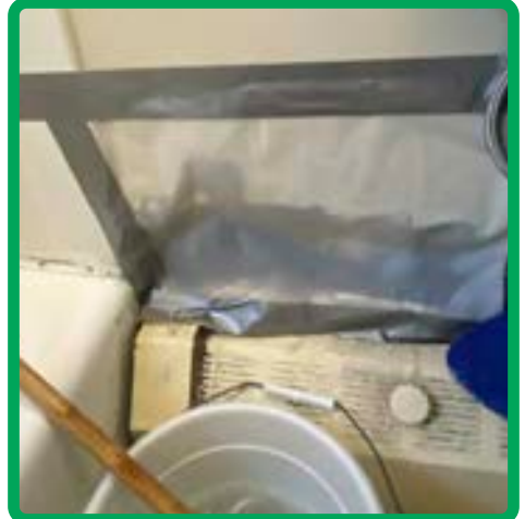
03: Hole in wall covered with tape and plastic by Maintenance
