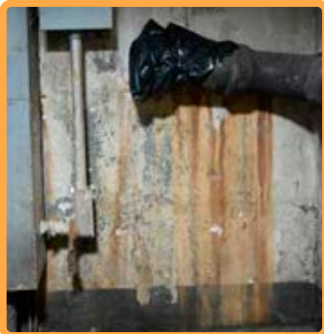
01: Leaking pipe main covered with garbage bag
