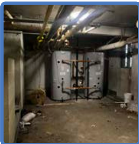
04: Recently installed hot water storage tanks in Tenant Storage
