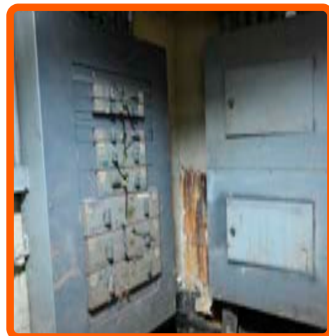
06: Electrical panels at end of useful life
