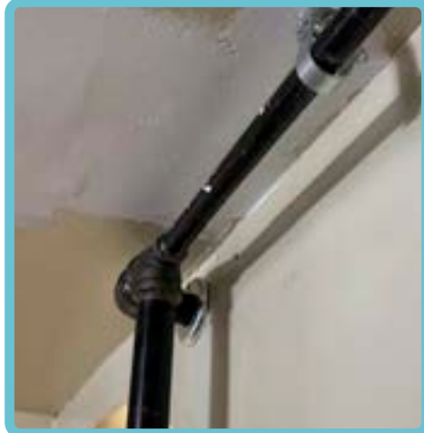
02: Retrofit gas pipe going through resident's living room
