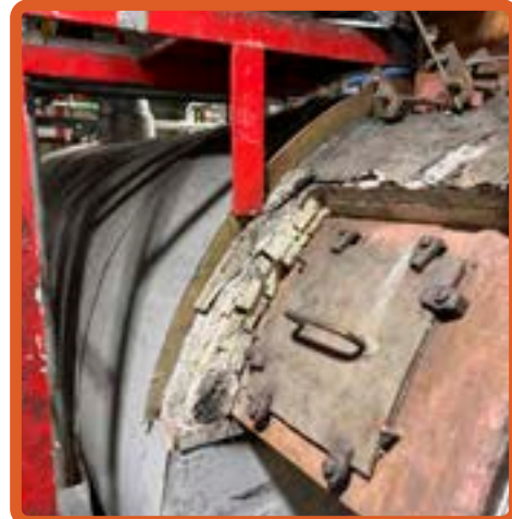
03: Existing boiler with corrosion; end of useful life
