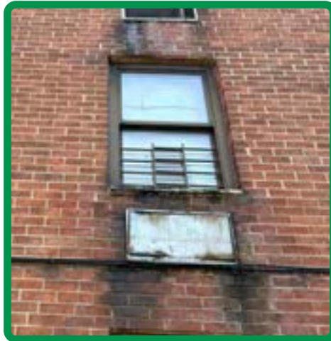
05: Deteriorating and mis-colored brick
