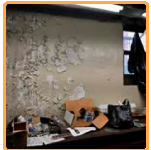
06: Water damage on foundation wall
