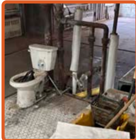
05: Apartment remains with existing end of useful life plumbing
